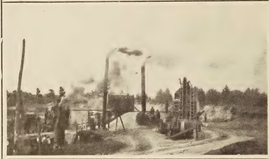
TOP: PORTABLE CRUSHING, SCREENING, AND DRYING PLANT. TEAMS ARE DRIVEN ACROSS PLATFORM AND RETURN. BOTTOM: SHOWING ROAD TO AND FROM CRUSHER PLATFORM. THIS IS A MORE ECONOMICAL ARRANGEMENT THAN WHERE THEY HAVE TO TURN ON THE PLATFORM.
