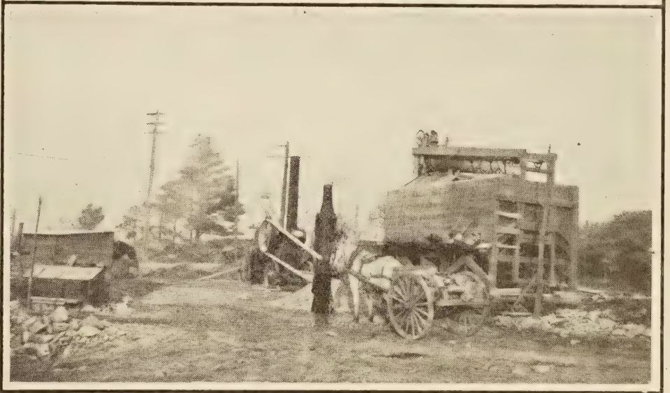
TOP: TEMPORARY QUARRY WITH TWO PORTABLE CRUSHING AND SCREENING PLANTS. DOWN GRADE TO HIGHWAY JUST TO LEFT OF QUARRY. BOTTOM: DELIVERING ROCK FROM TEMPORARY QUARRY NEARBY TO PORTABLE CRUSHING AND SCREENING PLANT FOR ROAD IN BACKGROUND.
