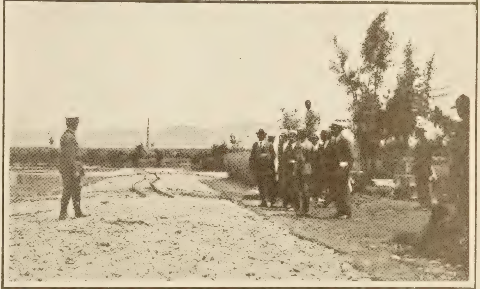
TOP: VIEW OF CONSTRUCTION WORK OF MODEL VILLAGE IN THE OUTSKIRTS OF PISA, ITALY, BY THE AMERICAN RED CROSS, LOOKING TOWARD THE CITY. BOTTOM: ROAD CONSTRUCTION IN THE MODEL VILLAGE.
