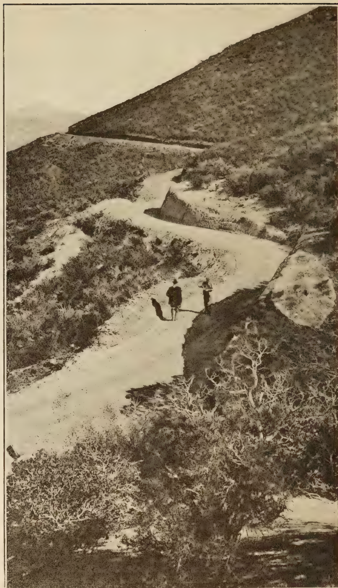
SECTION OF LAGUNA ROAD, CLEVELAND NATIONAL FOREST, CALIFORNIA. INEXPENSIVE TYPE OF CONTOUR ROAD.
