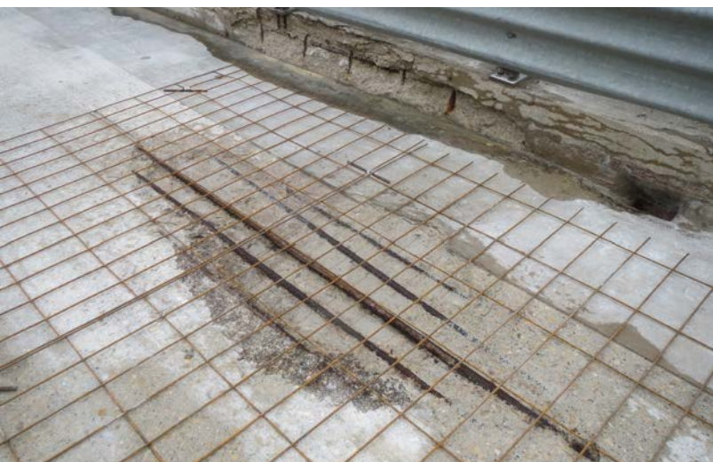
Before the bridge deck was rehabilitated, potholes exposed the deck's top reinforcement.
