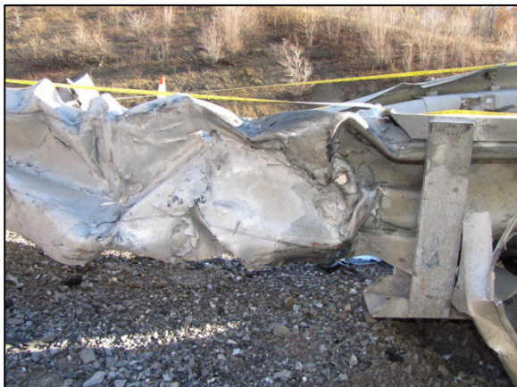
Figure 15: South-facing image of the buckled W-beam downstream of the end terminal.
