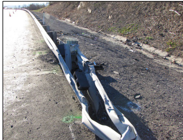
Figure 12: Northwest-facing view depicting the U-shaped deformed W-beam guardrail.
