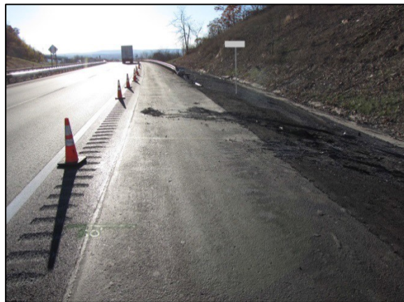
Figure 2: West-facing image approaching the crash site 15 m (50 ft) east of the point of impact.
