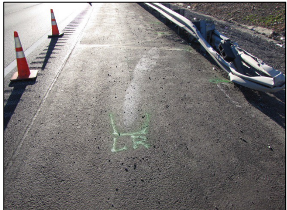
Figure 6: West-facing image depicting the left rear tire mark and deformed W-beam.
