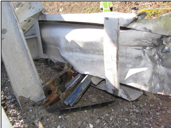
Figure 13: Northwest-facing image depicting the right (field) side of the end terminal and the end of the reinforcement bar in the feeder chute.
