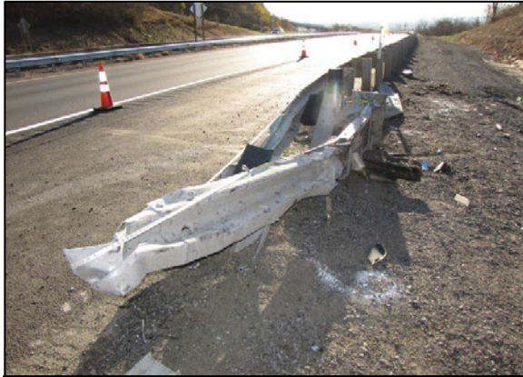
Figure 7: West-facing image depicting the U-shaped deformation of the W-beam between Posts 5 and 6.
