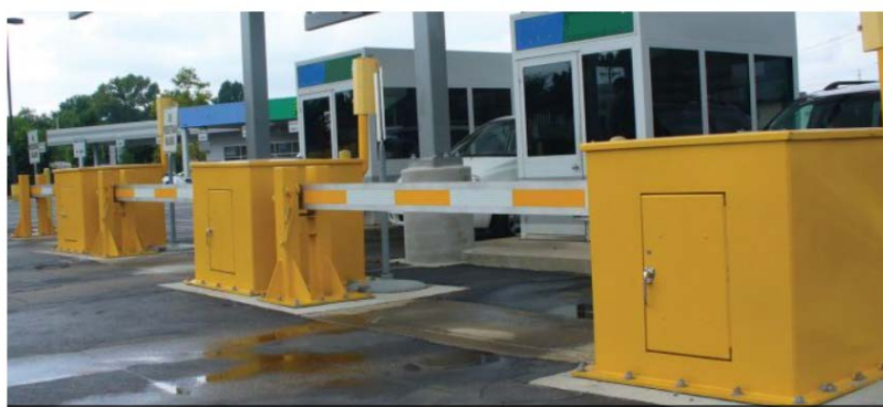
Figure 14. Photo. M30P1 active drop beam barrier—model M530.
