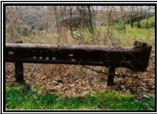
Figure 2. West view of struck W-beam guardrail.
